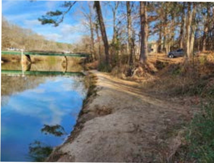
South River Existing Narrow and Eroding Embankment near Everett Park
